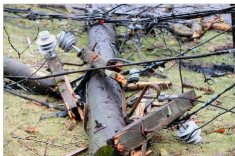
Storm damage in Westchester County, NY, March 12-15, 2010. Source: James Estrin / The New York Times
